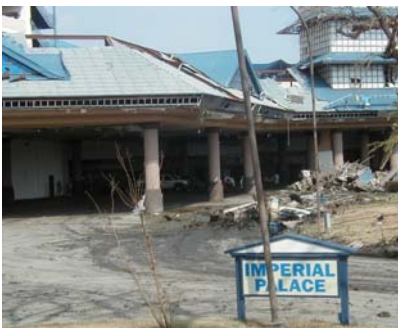
Main entrance was unusable
